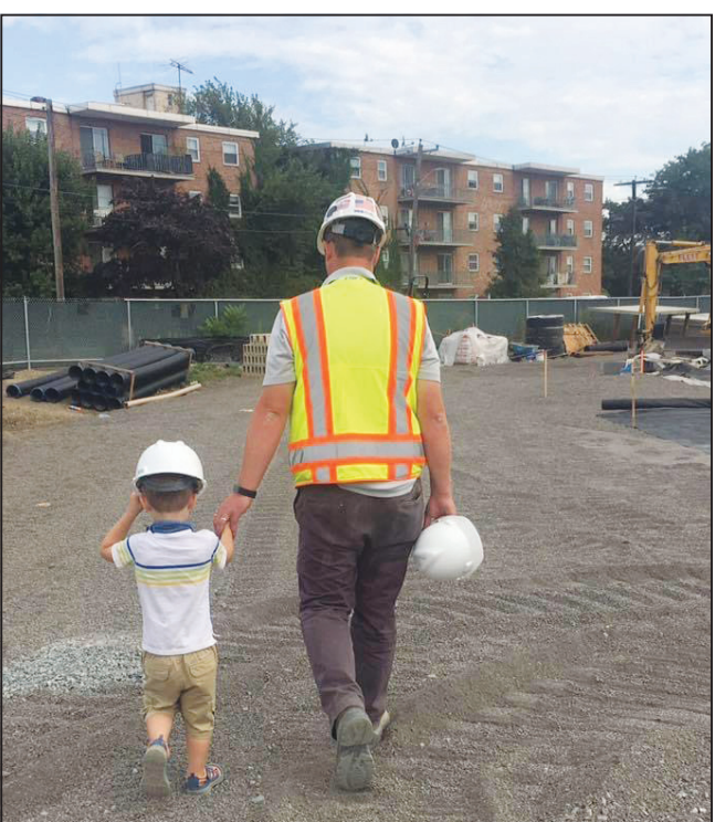
Miller Field Project Superintendent Matt Emanuelson walks with his son, Zach, in the early stages of the construction of the new field.
